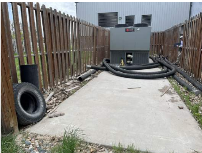
e. Image of damaged enclosure at
