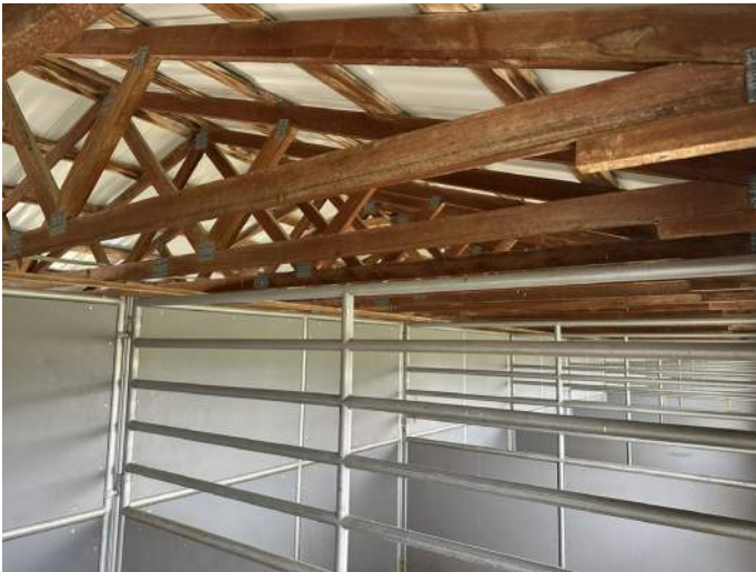
c. Image of pre-engineered wood truss and individual equine stalls. The Red Arrow identifies the exposed conductor noted in the narrative.
