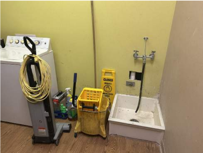
g. Image of the Laundry Room. Note the damage to the gypsum wall board above the mop sink. Also note the improper wall finish at this location.
