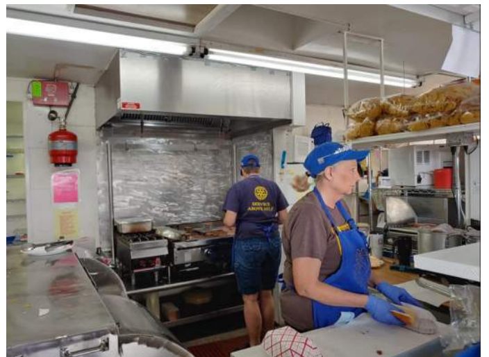
f. Image of the Rotary Kitchen with grill and commercial hood and ANSUL system in the background.
