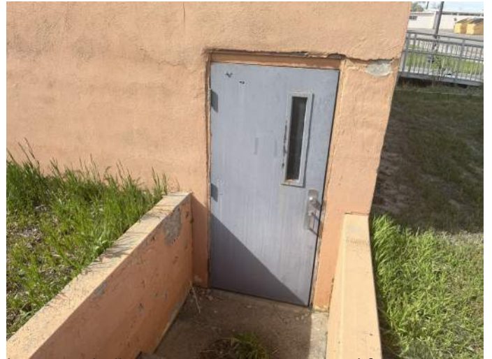
l. Image a hollow metal door set in a wood frame. The frame has rotted misaligning the door in the rough opening. The door is currently inoperable and is unable to open.
