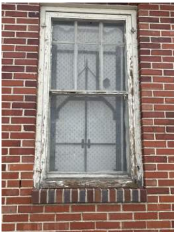
e. Image of typical single pane window with wood frame. Note the deteriorated condition of the wood frame. This is typical of all wood windows.
