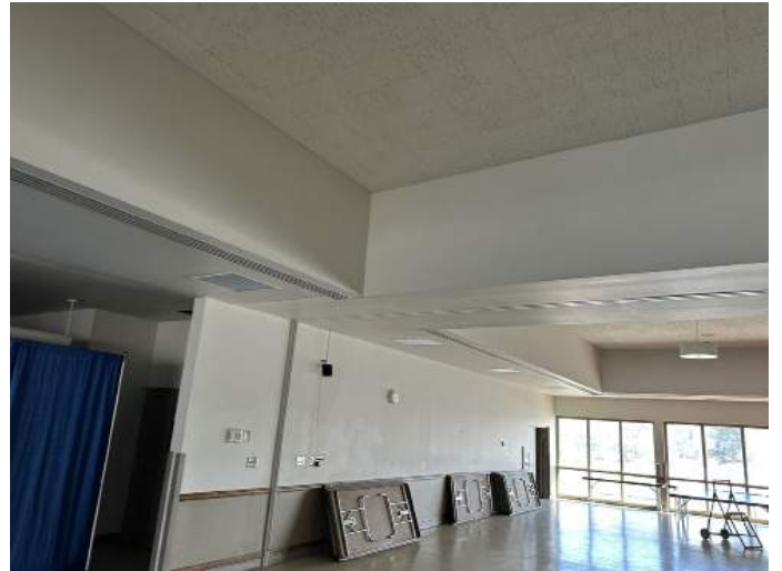
d. Image of the Multi-Purpose Space within McKibben Cafeteria. Note the paint finish on the gypsum wall board. It appears this wall should be re-painted in its entirety.
