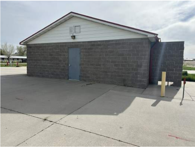
g. Image of damaged rain gutter and fascia.
