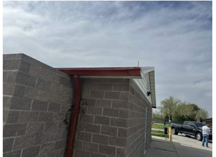
b. Image of damaged rain gutter.
