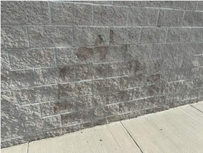
a. Image Split face CMU block spalling at exterior wall of building.
