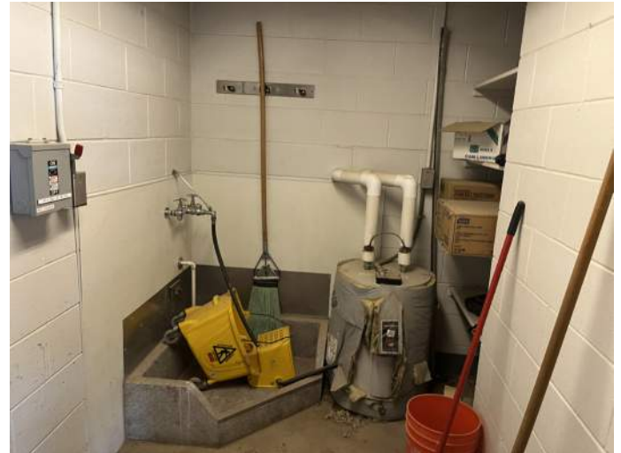
d. Image of the mop sink and hot water heater in one of the Custodian Closets.
