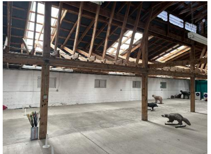
d. Image depicts the post and beam framing structure complete with skylights and clerestory louvers.
