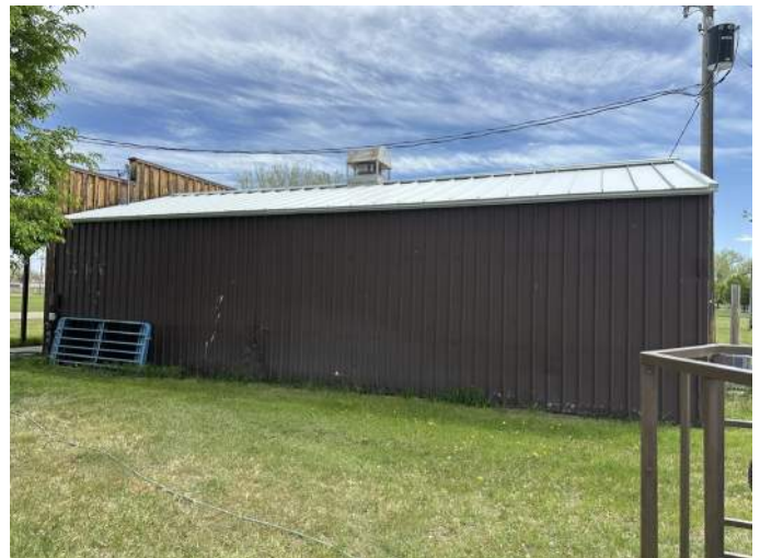
d. Image depicting damage to the PEMB metal wall panel.
