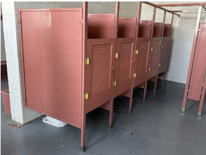
k. Image of the mop sink and one of the lavatories that appear to be original fixtures to the building. Note - The fixtures are non-functioning.
