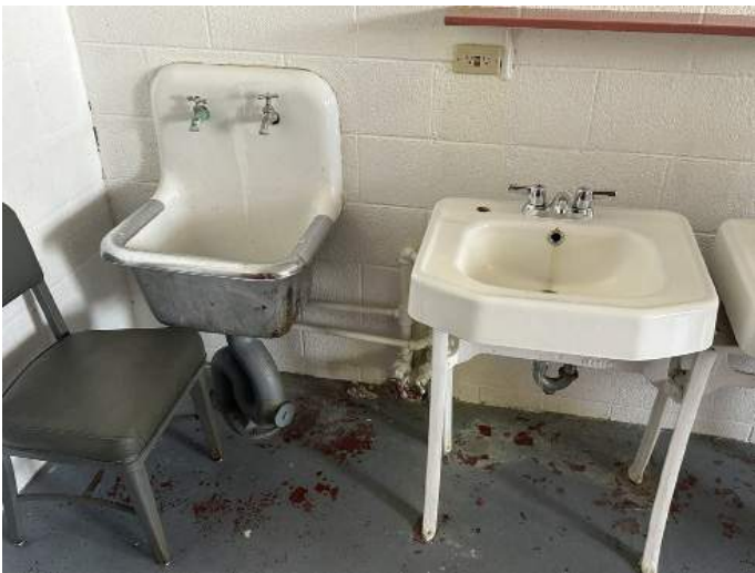
i. Image of the mop sink and one of the lavatories that appear to be original fixtures to the building. Note - The fixtures are non-functioning.
