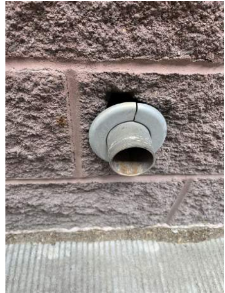
b. Image of CMU block that requires repair in order to keep out pests and the elements.
