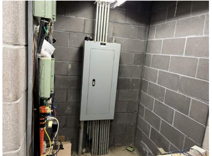
h. Image of Electrical Panel.
