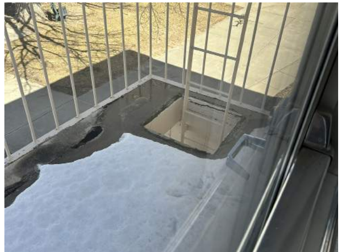
d. Image of the crumbling concrete at the fire escape and the fire escape ladder and access hatch.
