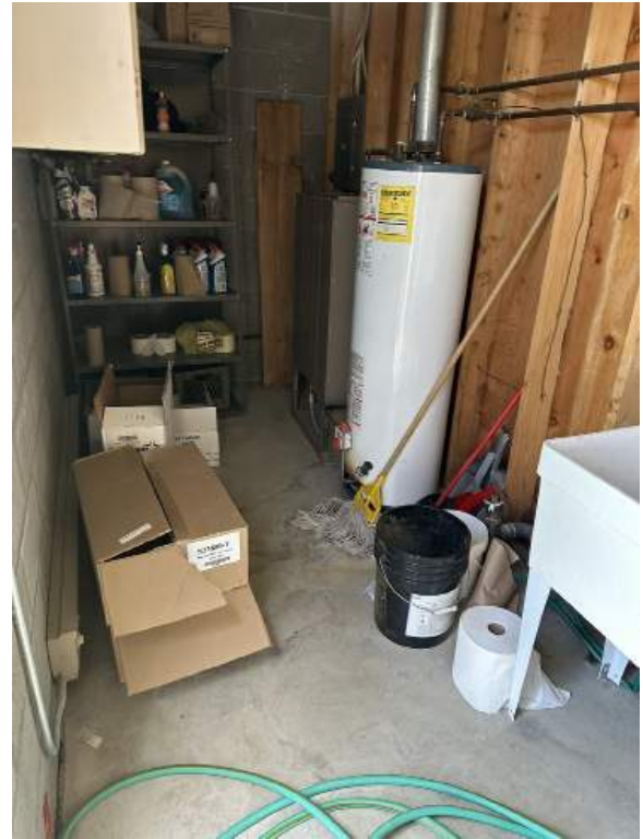
g. Image of the plumbing chase between the restrooms depicting hot water heater, and electrical panel.
