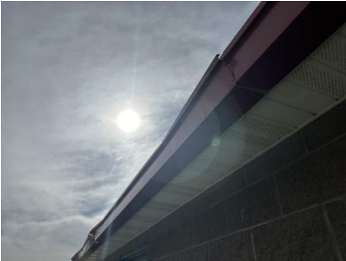
a. Image of damaged rain gutter.
