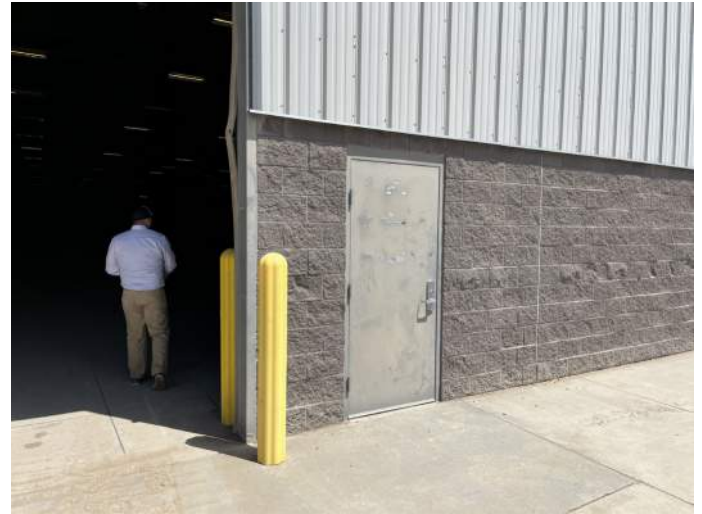
b. Image of damaged side seal at sectional overhead door on the South side of the building.
