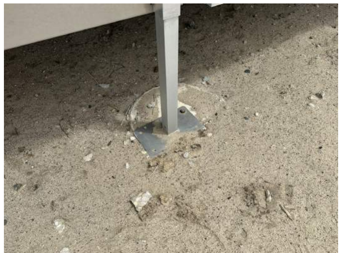
f. Image of concrete foundation with off centered base plate for the aluminum ramp system. Note, the base plate is only attached with a single fastener.
