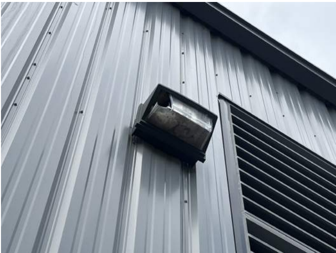
c. Image of damage to the lens of an exterior wall pack.
