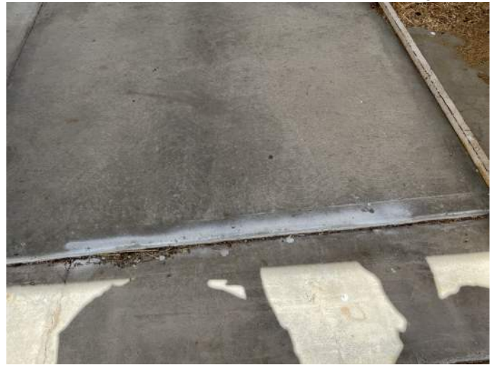
d. Image of the change in level along the accessible route that exceeds the standards for accessible design.
