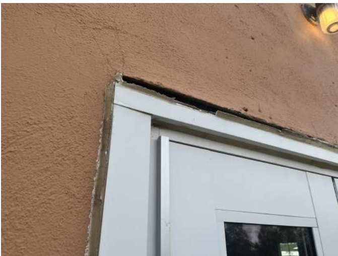
g. Image taken at the head of the aluminum storefront door. Note the sealant has completely failed allowing the elements into the wall and building.
