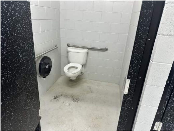
g. Image of the accessible water closet. Note the flush handle is on the wrong side of the tank.
