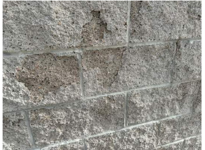
b. Close up image of spalling split face CMU block noted in Image a.
