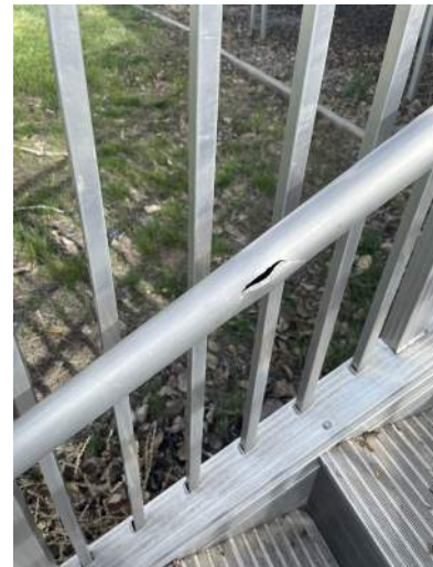
n. Image of damage to the handrail on the North Elevation facing Fort Reno. This is hazardous to patrons as it has the potential to catch a ring, or article of clothing.
