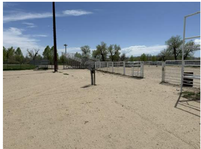
f. Image depicts metal junction box in open area.
