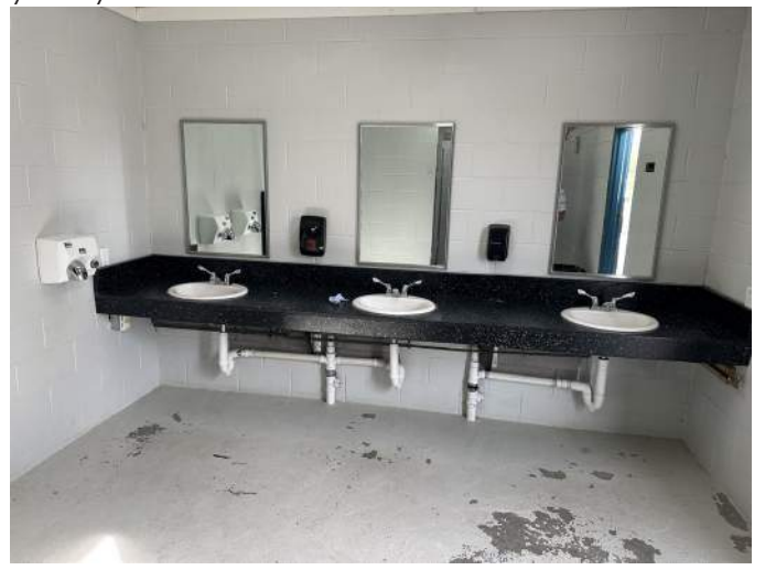
f. Image of lavatory. Note the thermostat under the counter on the left hand side of the image and the wall hydrant on the right hand side of the image.
