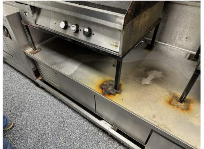
f. Image depicts standing water adjacent to the cook top and fryer as well as a shim type system that does not comply with the kitchen equipment manufacturers installation instructions. The kitchen should be upgraded to comply with modern codes and standards.
