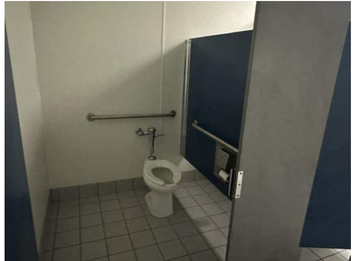
n. Image of the Wheel Chair Accessible Toilet Compartment in the Men's Restroom. Note the flush control faces the wrong direction.
