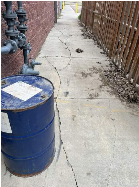
i. Image of cracked concrete at between East facing elevation at the mechanical equipment enclosure.
