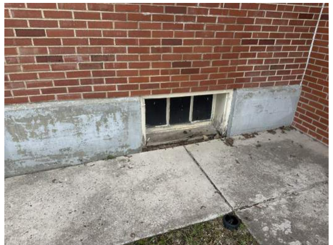
f. Image of typical single pane window with wood frame at grade. Note the deteriorated condition of the wood frame and window glazing. This is typical of all wood windows at this location.
