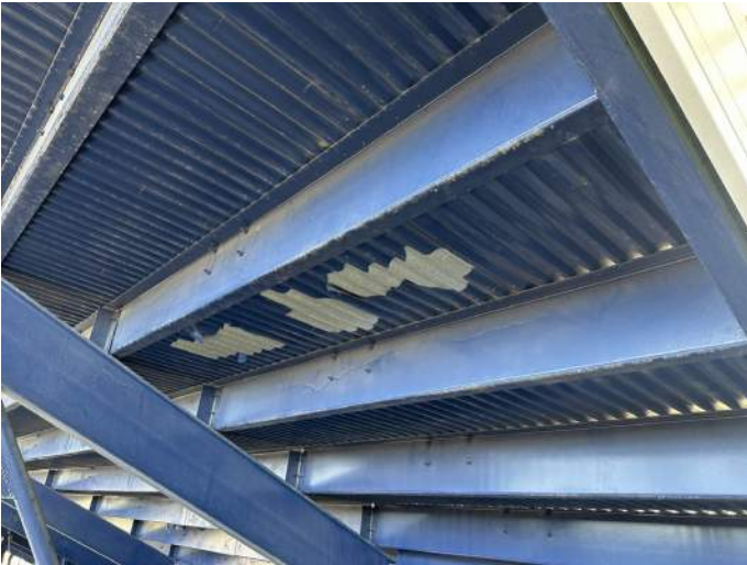
a. Image depicts paint peeling from underside of the Grand Stand structure.
