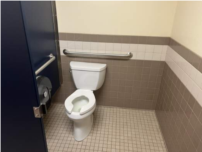
u. Image of the wheel chair accessible toilet stall in the Women's Restroom. Note the flush handle is on the wrong side of the tank and needs to be changed to the other side.
