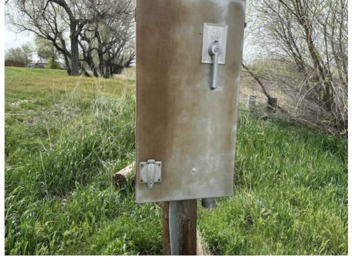
o. Image of disconnect switches open to public access and spaces. It is not know if the disconnect in the image are active and functional.
