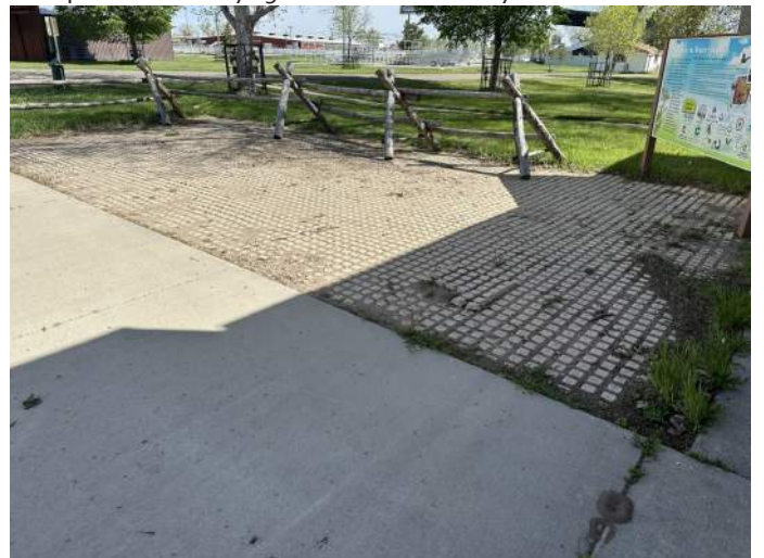
f. Image depicts a cobbled patio space. This is not ADA accessible.
