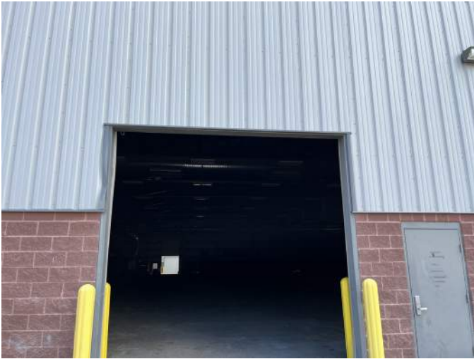
g. Image of damaged metal trim at the jamb of the sectional overhead door.
