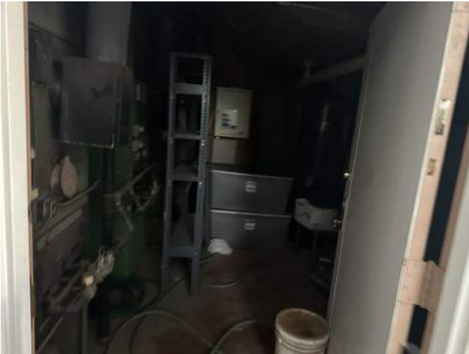
s. Image of the electrical panel in the Mechanical Equipment Room.
