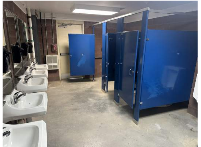
t. Image of conflict of exterior door and toilet partition.
