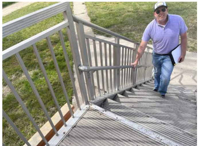
h. Image of the handrail at the stair on the North facing elevation of the building. Note the height of the handrail shall be not less than 34" and not more than 38."
