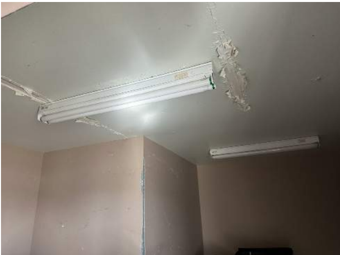
e. Image of damage to the gypsum board ceiling in the Storage Room due to a roof leak.
