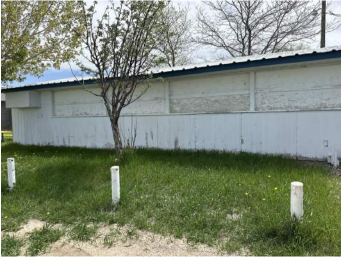
i. Image of TI-II plywood siding panels. Notice the paint finish beginning to fail, the relationship of the siding panel relative to grade and the condition of the wood, and the visible location of the fasteners.
