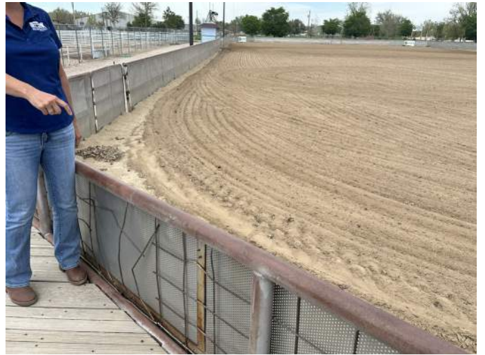
d. Image of damaged welded wire fence panel. This panel poses a tripping and snagging hazard.
