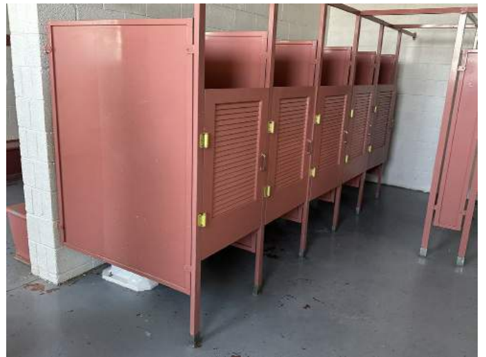
j. Image of the toilet compartments. Note - The waterclosets are non-functioning.
