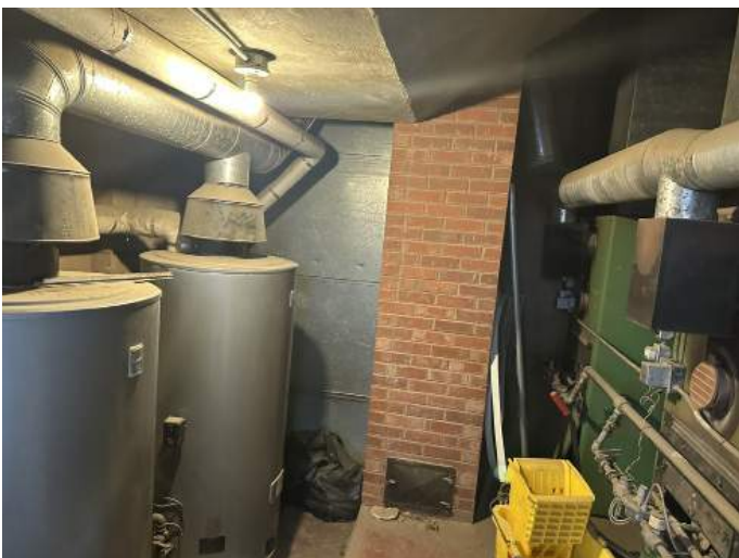
q. Image of the interior of the Mechanical Room on the Ground Floor.
