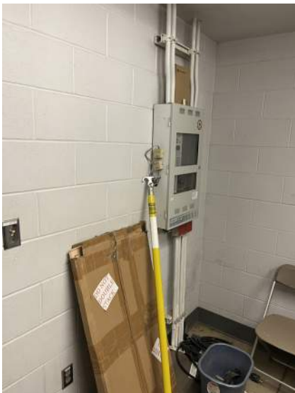
k. Image of Fire Alarm control panel in one of the pavilion offices.
