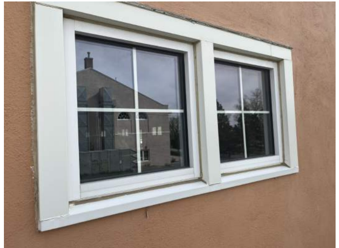
f. Image of a new vinyl window. Note the exposed wood at the head of the window and sealant which has peeled away.
