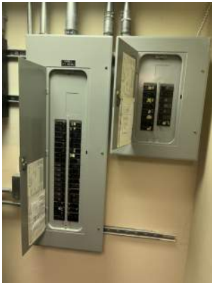
m. Image of the interior of the Furnace Closet on the Ground Floor / Main Level.
