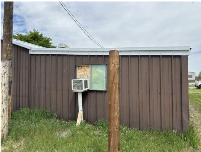
c. Image depicting the existing aluminum window, the window mount condensing unit and support.
