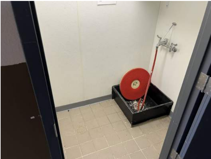
s. Image of the interior of the Utility Closet.
