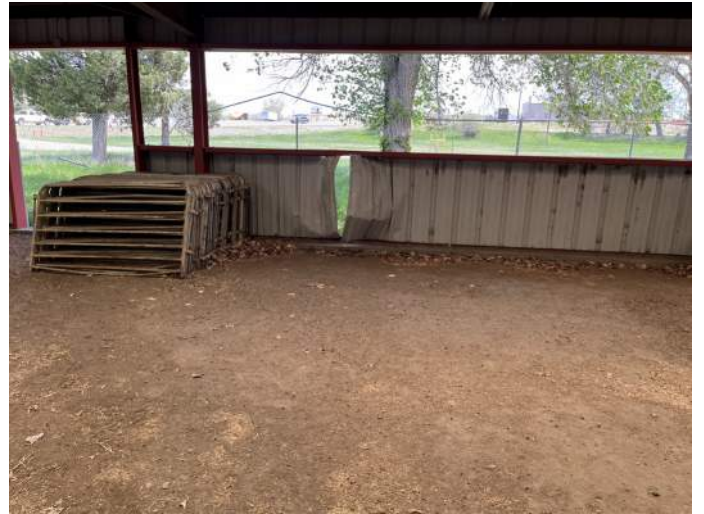
b. Image of damaged metal wall panel looking East.
