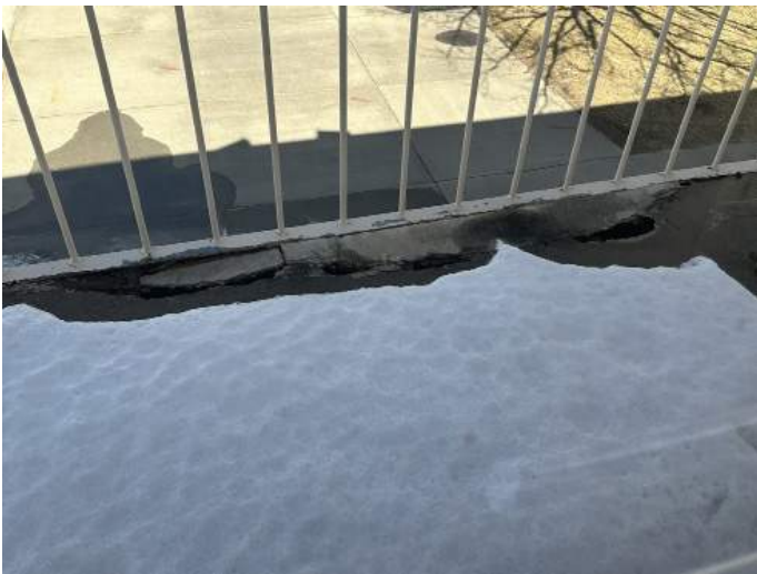
c. Image of the crumbling concrete landing at the fire escape.
