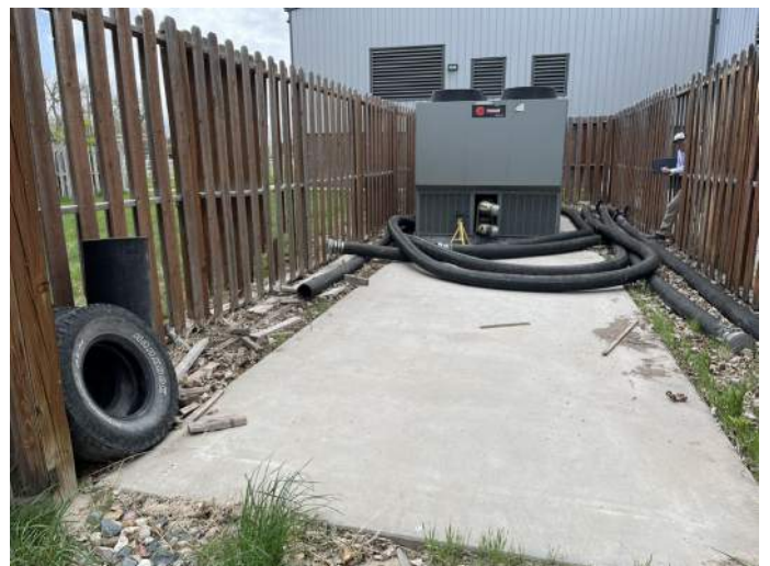
f. Image of damaged enclosure at
