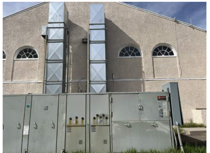
p. Image of the ground mounted packaged air unit.
