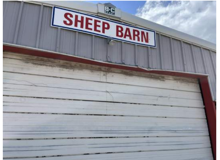
d. Image of damaged head and cover trim and side seal at the sectional overhead door.
