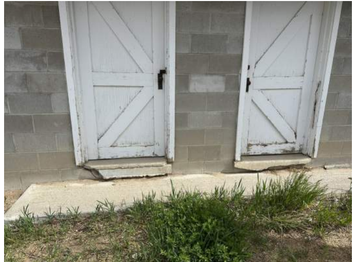
j. Image of additional exterior doors to tack and storage rooms at Stall Barn 'B'. The Red Arrow identifies where the concrete spilled out to the exterior when the interior slab for the tack and storage rooms was poured. This condition poses a tripping hazard and should be removed.
