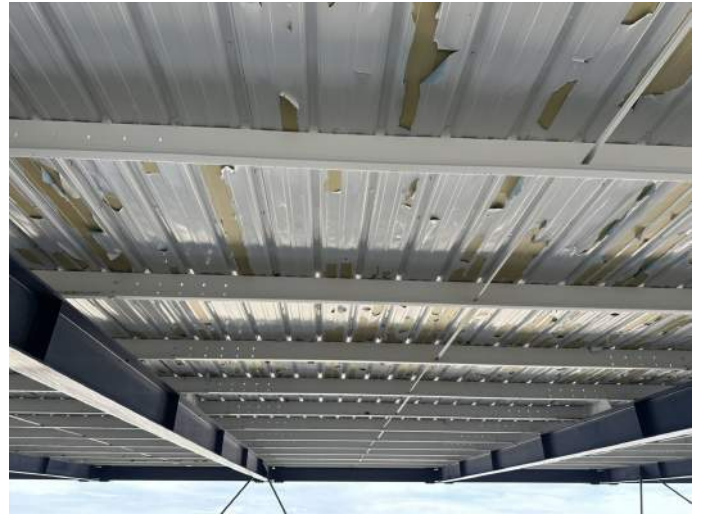
b. Image depicts paint peeling from the soffit of the roof over the tiered seating.
