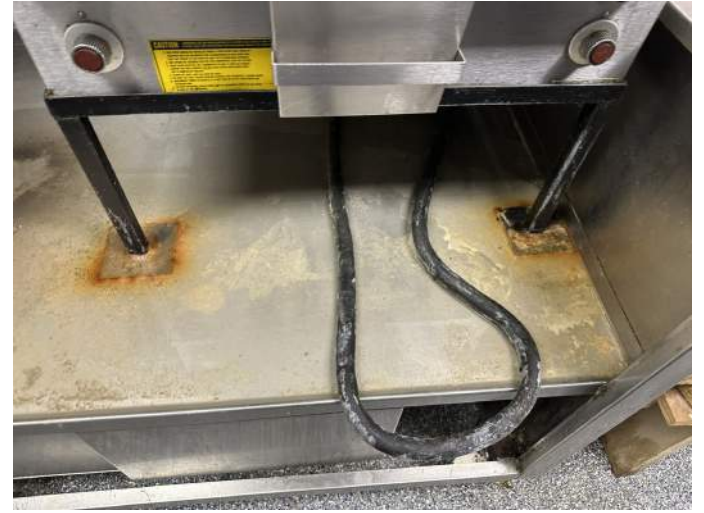
h. This image illustrates the presence of standing water beneath the fryer, as well as the positioning of a power cord in an area where it is susceptible to being snagged.
