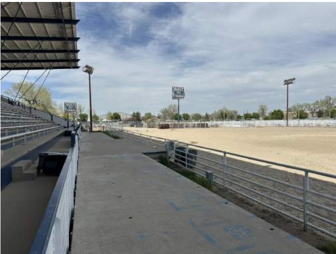
c. Image depicts the existing podium/walk way in front of the grand stands. The required guard rails are missing along the length of the podium.
