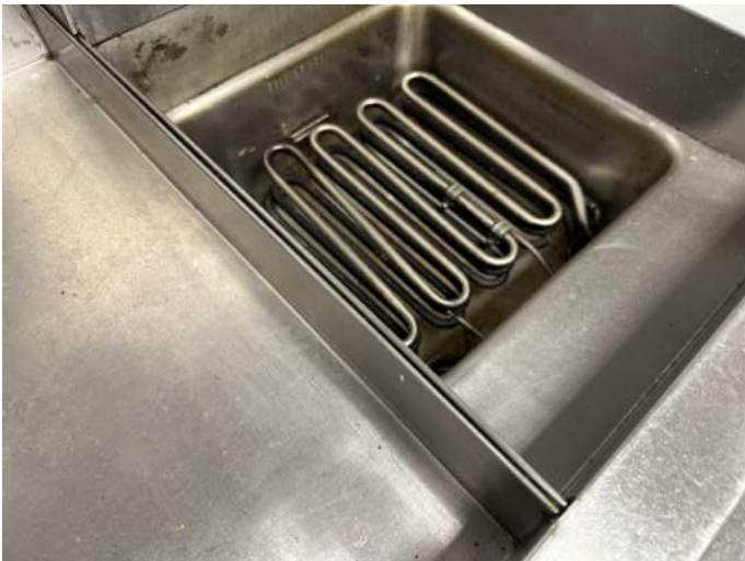
g. Image depicts standing water in the heating element for the fryer.
