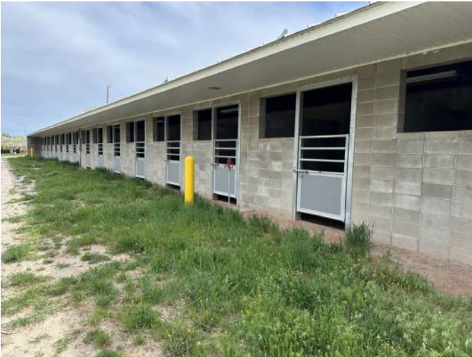
l. Exterior of the stalls at Stall Barn 'F' as viewed from the South.
