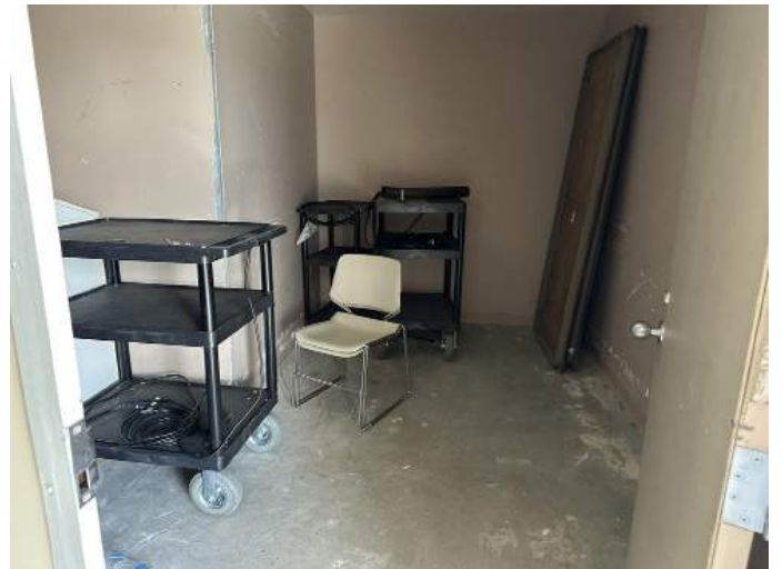
f. Image of damage to the interior walls of the Storage Room.
