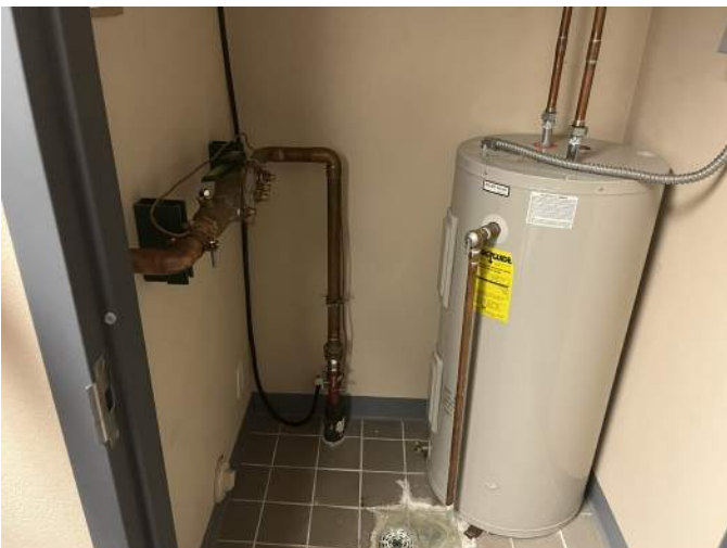
i. Image of Hot Water Heater storage closet.
