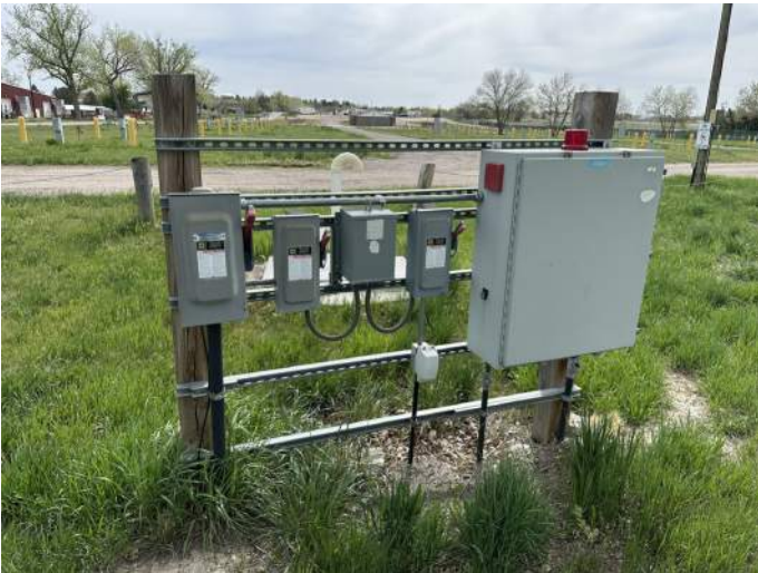
n. Image of disconnect switches open to public access and spaces.
