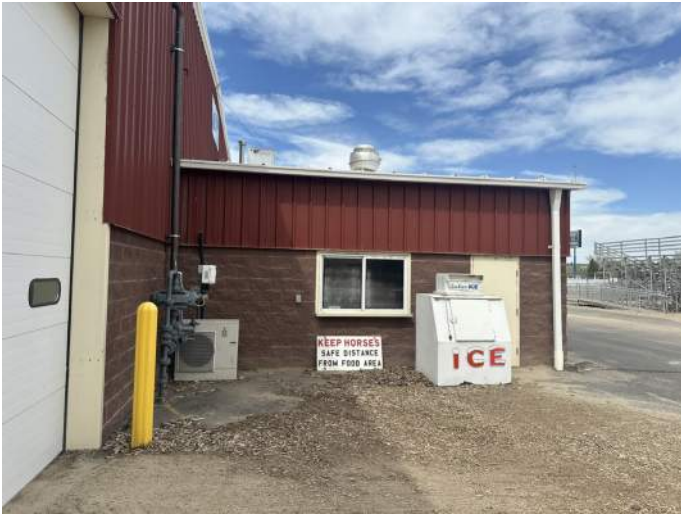
u. Image of proximity of outdoor unit for mini-split system to the natural gas riser.
