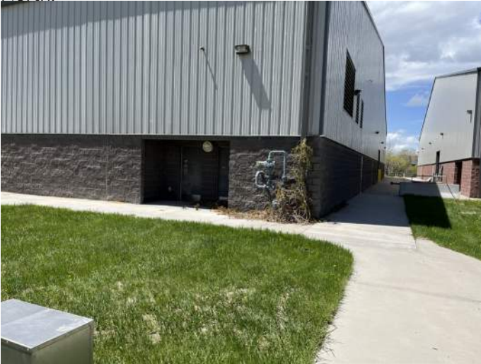
i. Image of commercial gas meter and rain gutter downspout with vines growing and overtaking both.
