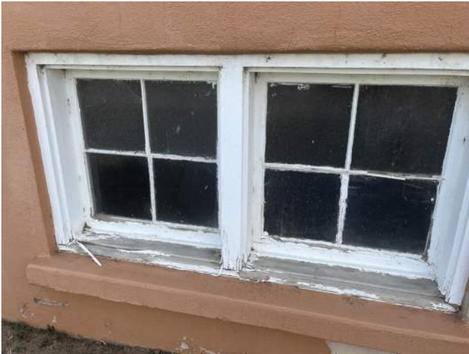
k. Image of typical wood window. Note the window glazing has failed and is falling off of the window.
