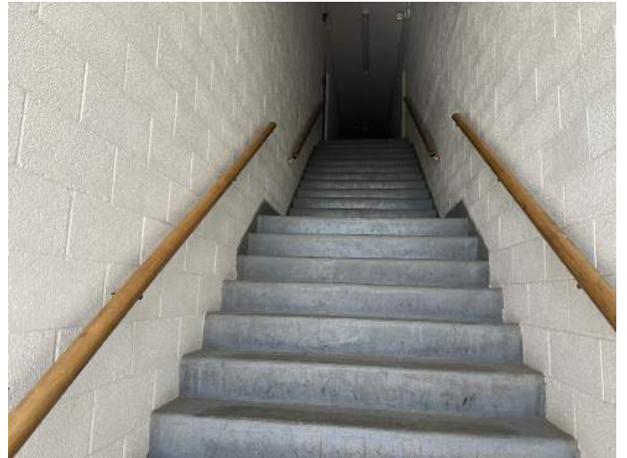
n. Image of the Stair leading from the exterior of the building at grade to the Upper Level.
