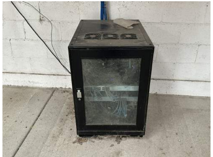
l. Image depicts the server cabinet for the Vyve building.
