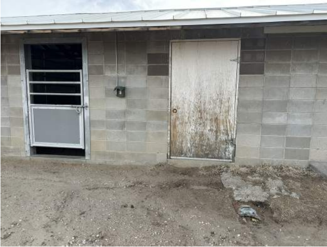
g. Image of wood door and frame, and clogged storm drain.
