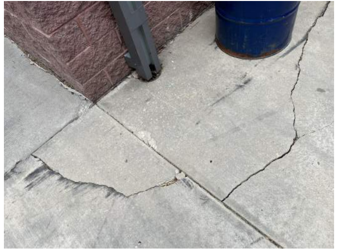
h. Image of cracked concrete at downspout.
