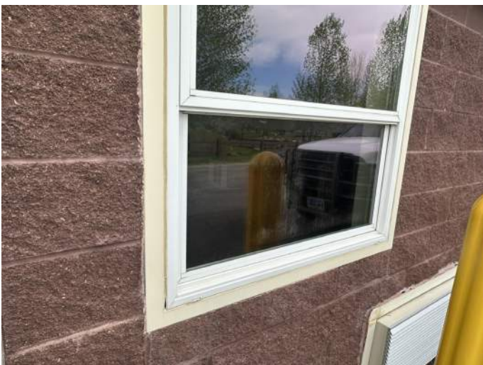
w. Gaps at sealant at windows and PTAC.
