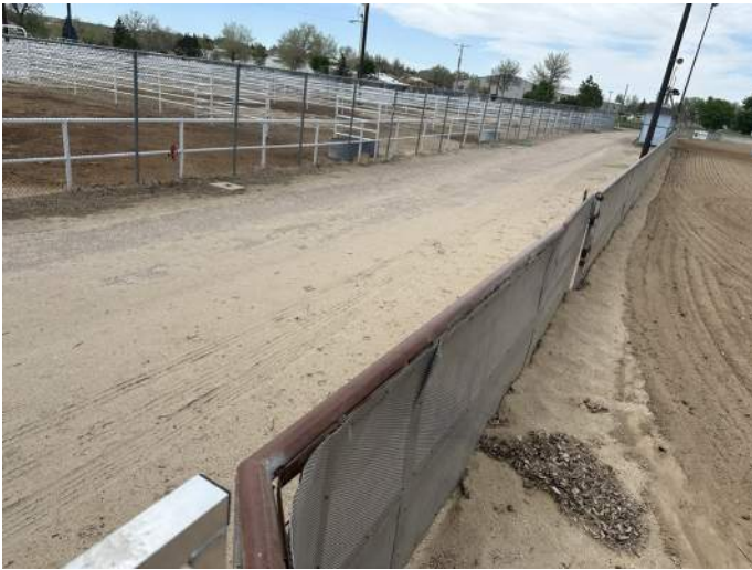
c. Image of damaged perforated aluminum panel .
