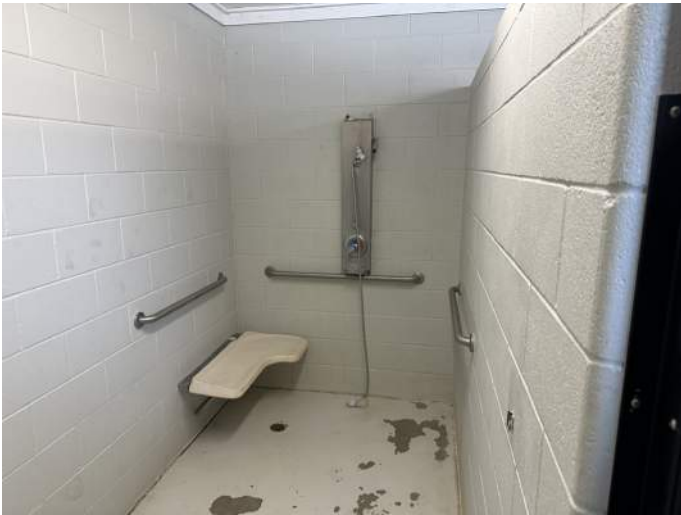
c. Image depicts paint peeling from shower floor.
