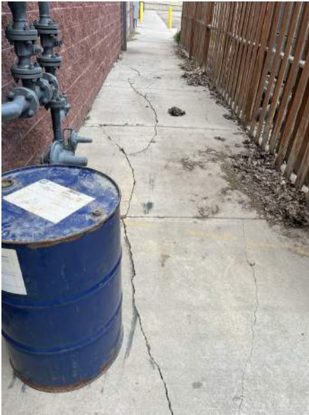
a. Image of 55 gallon oil drum adjacent to the gas meter.
