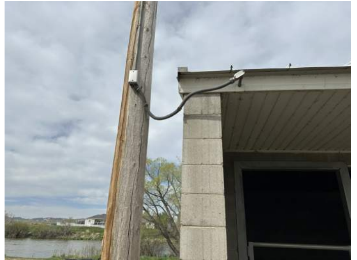
m. Image of power drop on the South side of Stall Barn 'F'.
