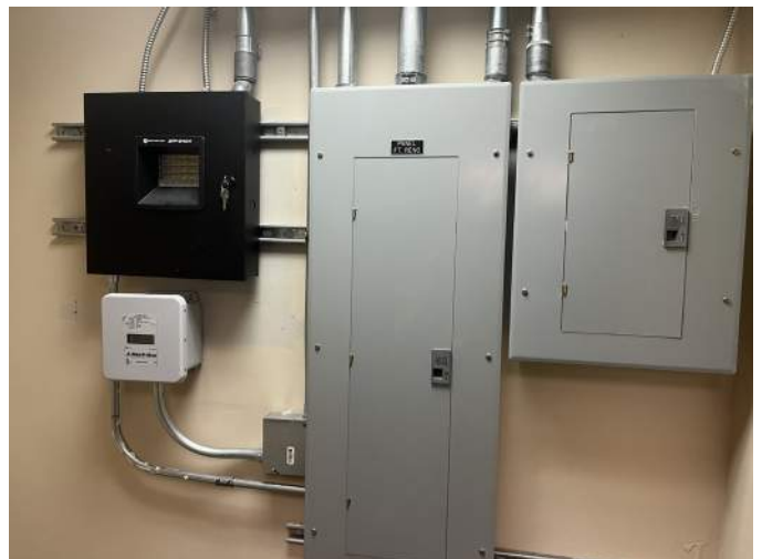
j. Image of Electrical Panel and Fire Alarm Control Panel.
