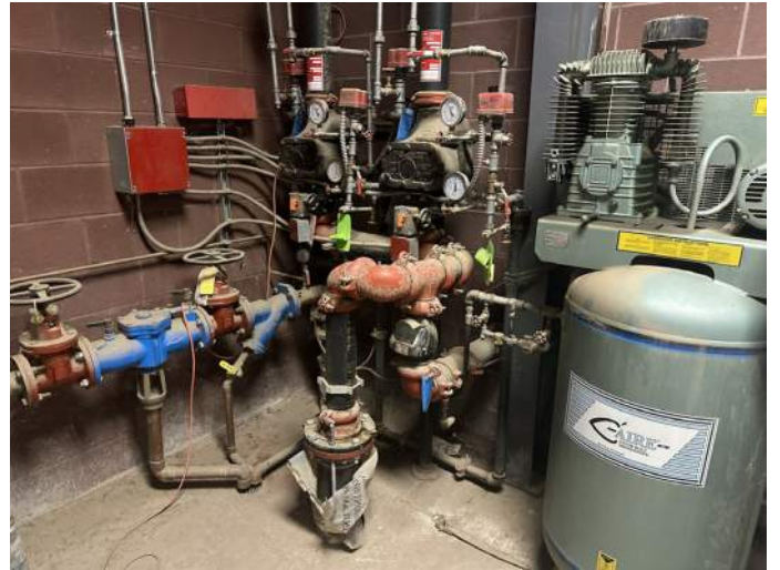
v. Image of air gap at floor drain.
