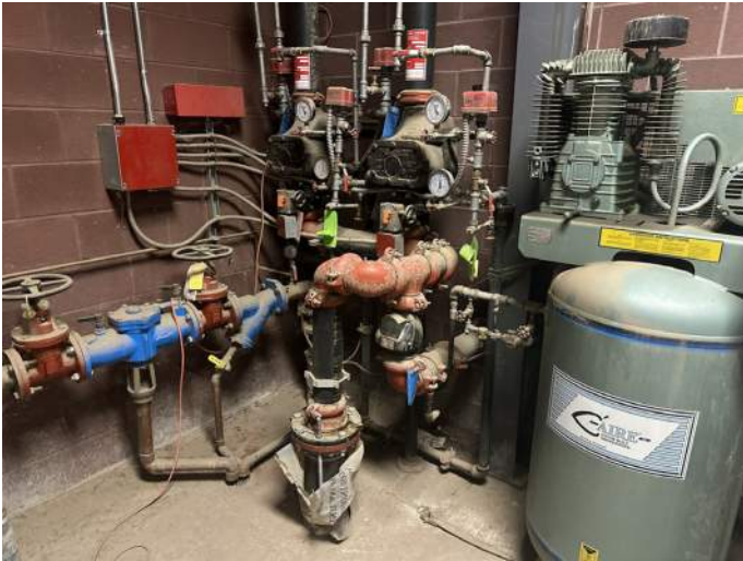
s. Interior Image of Mechanical Room.
