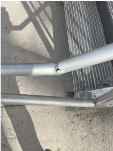
m. Image of damage to the handrail on the North Elevation facing Fort Reno. This is hazardous to patrons as it has the potential to catch a ring, or article of
