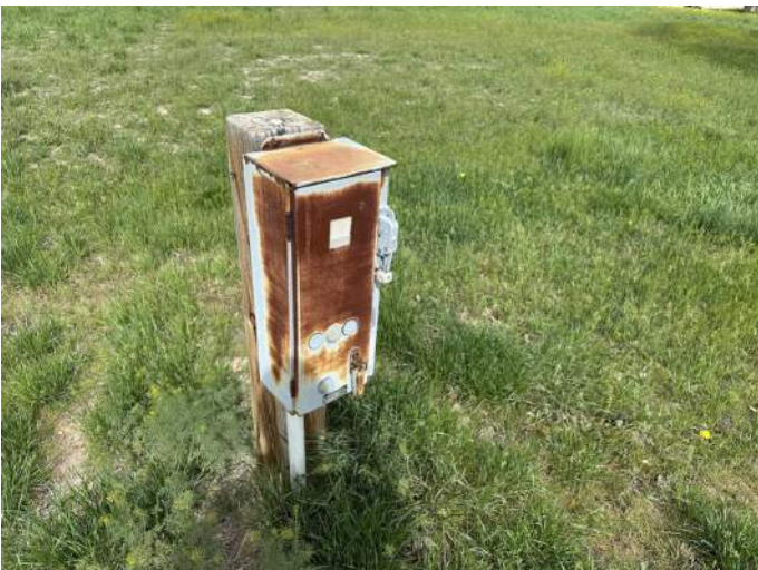
p. Image of disconnect switches open to public access and spaces. It is not know if the disconnect in the image are active and functional.
