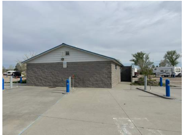
d. Image the exterior of the North Elevation. Note the split face CMU block face is spalling just behind the yard hydrant.
