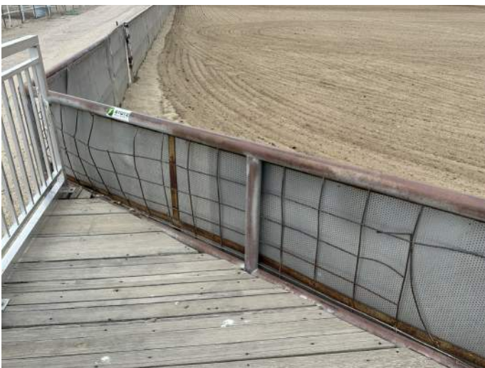
e. Image of damaged welded wire fence panel. This panel poses a tripping and snagging hazard.
