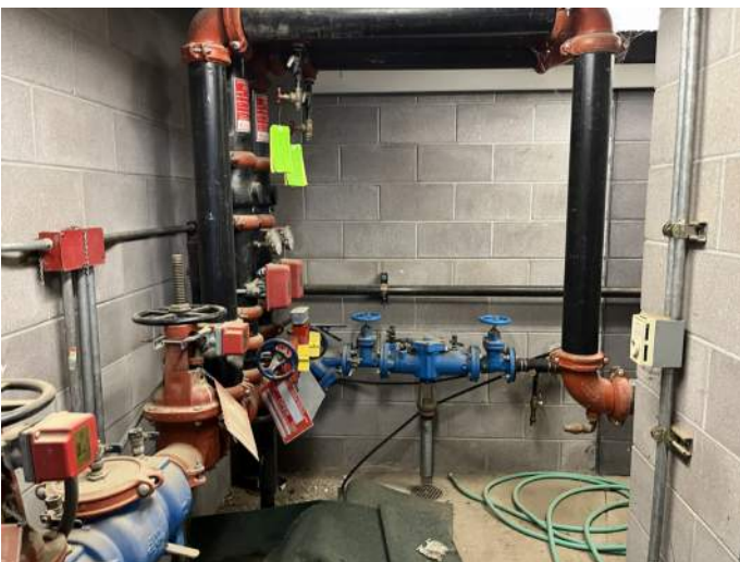
e. Image of the Fire Riser.
